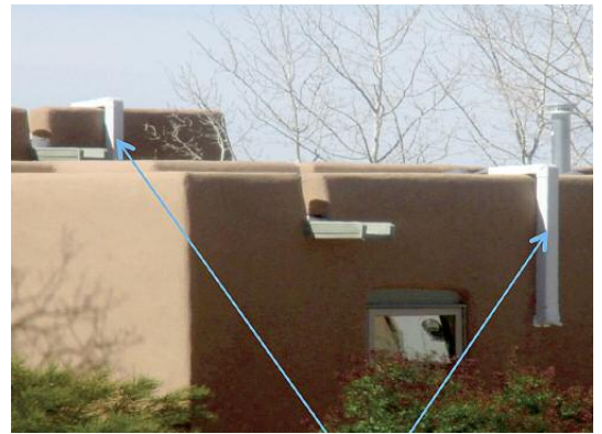
Arrows indicate white-painted ducts.
